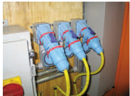
Typical load station in Stolle plant is equipped with multiple Decontactors to facilitate testing and customer runoff of new machinery.
