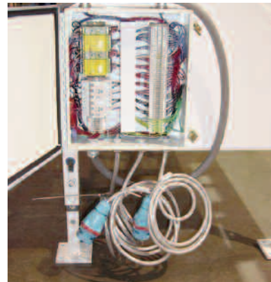
An auxiliary control panel and related equipment can be safely connected and disconnected to the mating Decontactor receptacle on the shell press.
