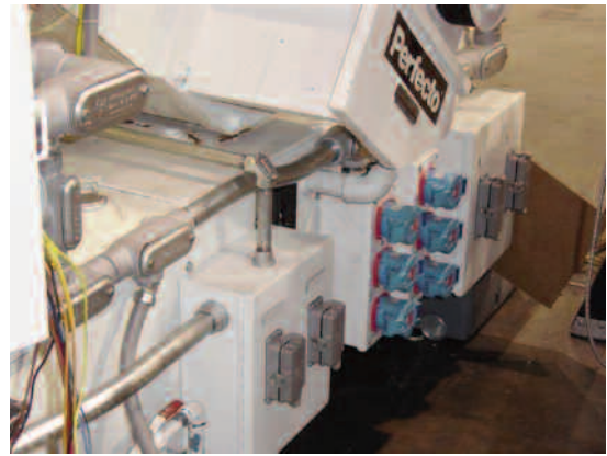
Switch rated Decontactor receptacles are used to connect power from a shell press to auxiliary equipment.
