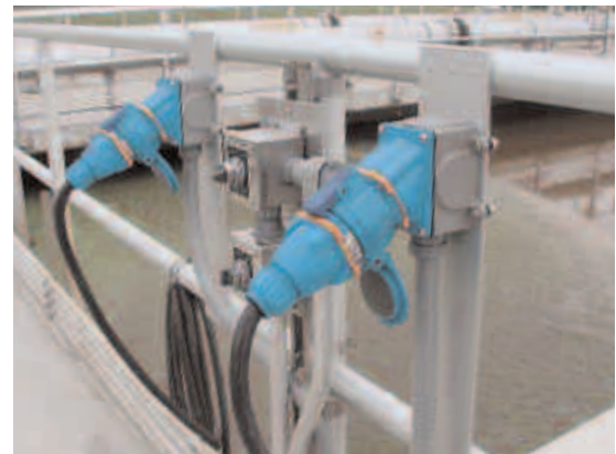
Closeup shows Meltric Decontactors for two adjacent mixers. Pressing the pawl on top of the device disconnects the power safely before the plug and receptacle can be separated.
