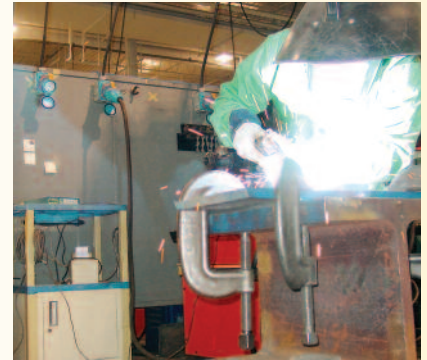
Switch rated welding receptacles (background) are connected to overhead busway system via cord drops.
