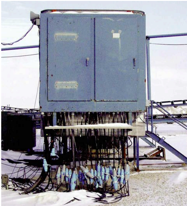
In-line connections are preferred at this quarry to solve a mounting space problem.
