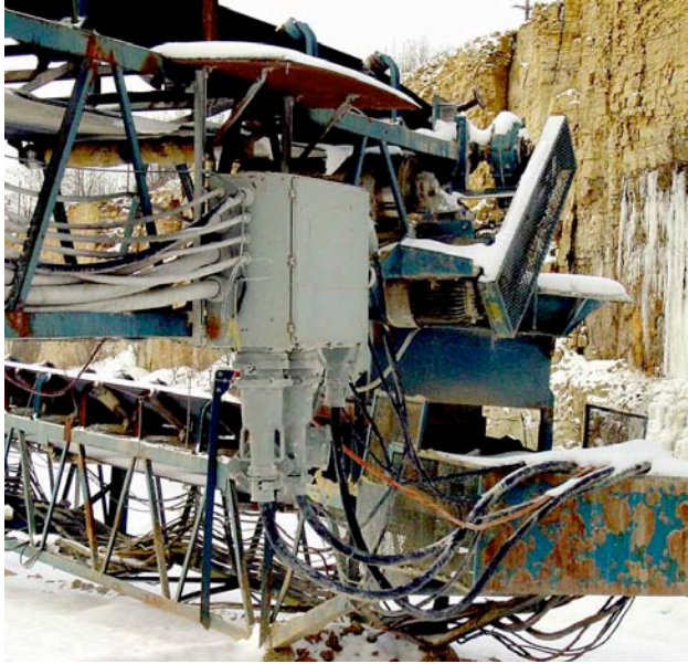
Power to a 500 horsepower crusher motor is supplied by parallel phasing of two 400A PF plugs and receptacles.
