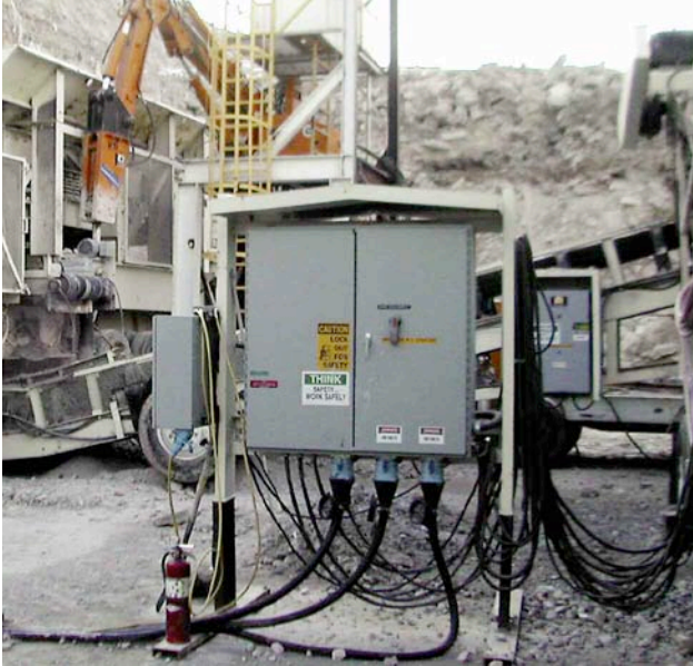
200A DS200's distribute power from portable generators to a power distribution panel (pictured) and then to conveyors and other electrical equipment. A DSN24 Multipin connector (left of the panel) provides control wire connections to the PLC cabinet in a single convenient connector.
