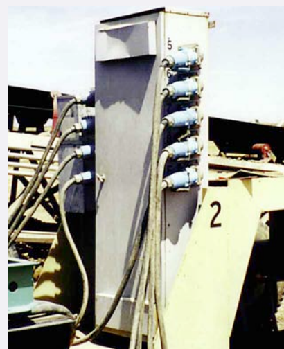
Mobile power distribution panel
