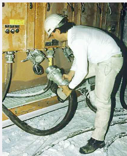
Mobile generator at salt mine
