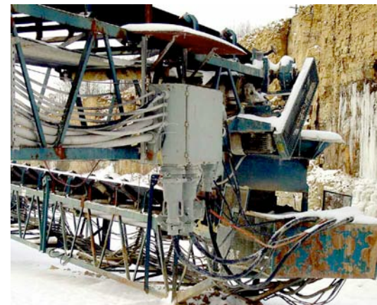
PF devices provide power to a 500 hp crusher motor
