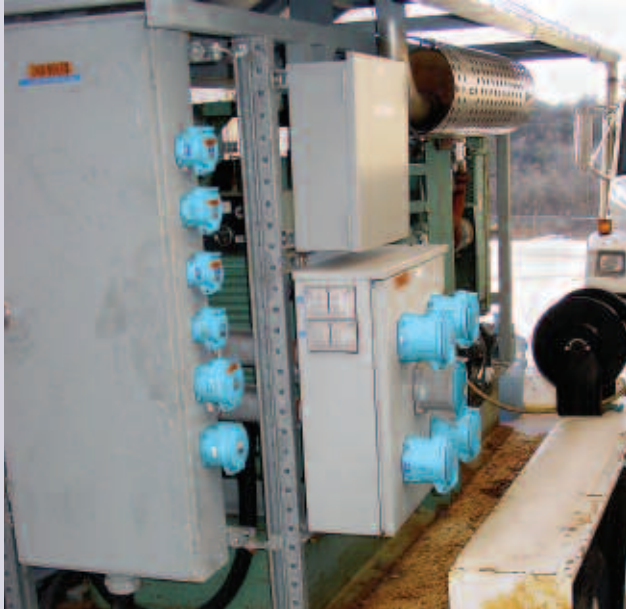
A mobile diesel generator supplies power via Meltric plugs & receptacles during outage conditions.
