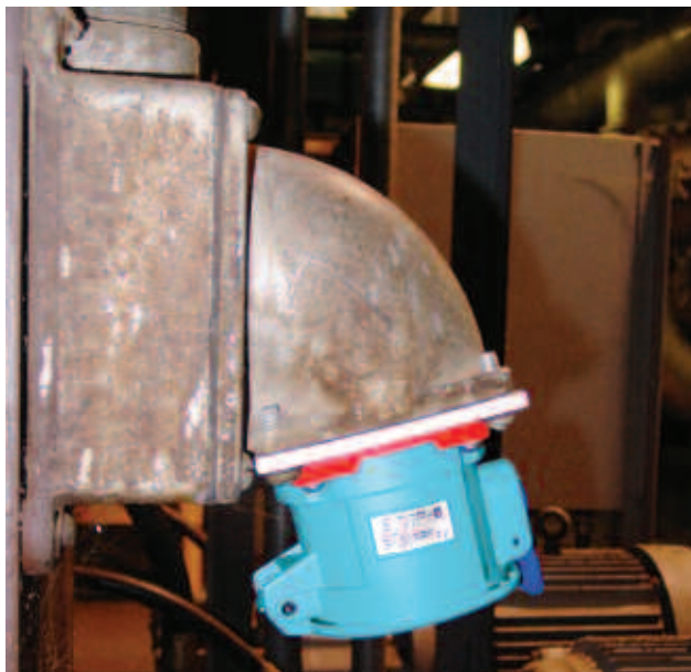
Adapter plates made it simple for this power plant to convert their existing pin and sleeve receptacles to Deconnectors.
