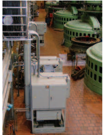
Power Receptacles (lower left)
