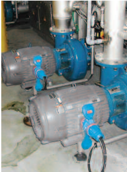
Process Pump Connections
