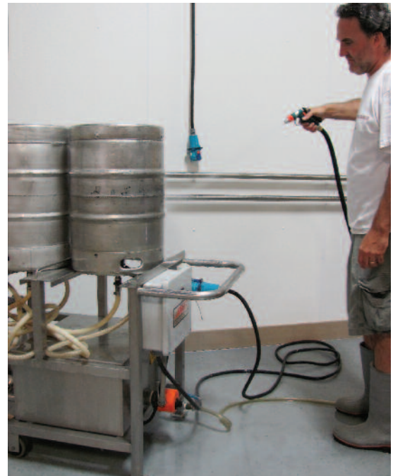
Washing down equipment is a frequent activity at the House of Brews. The Meltric Decontactor Plugs and receptacles are automatically NEMA 4X watertight whenever they are mated together.
