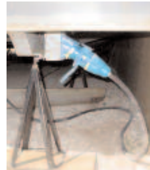
A male inlet is installed at the mobile classroom corner opposite the panel. The female connector is easily mated to the inlet providing a safe and neat power connection.
