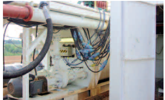
Pumps and other equipment are also connected.
