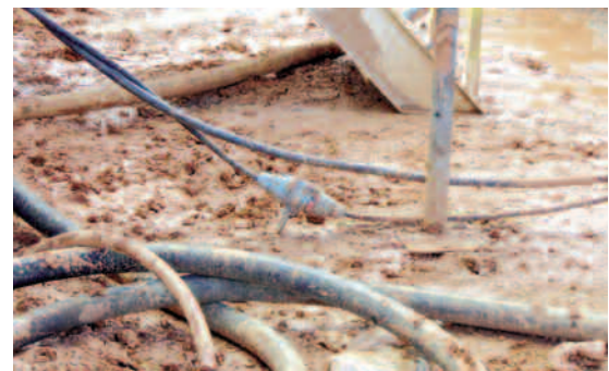
Adverse conditions include water, mud and temperature extremes, yet the Deconnectors have continued to operate reliably since being installed.
