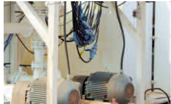
Electrical motors that operate on 440 VAC are among the equipment connected with the Deconnectors, which can be seen above.
