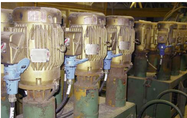
Decontactors enable quick motor change-outs
