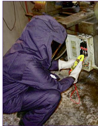
After operating the disconnect switch, a worker still needs to verify deenergization. Exposure to live parts is inevitable, so PPE is required.
