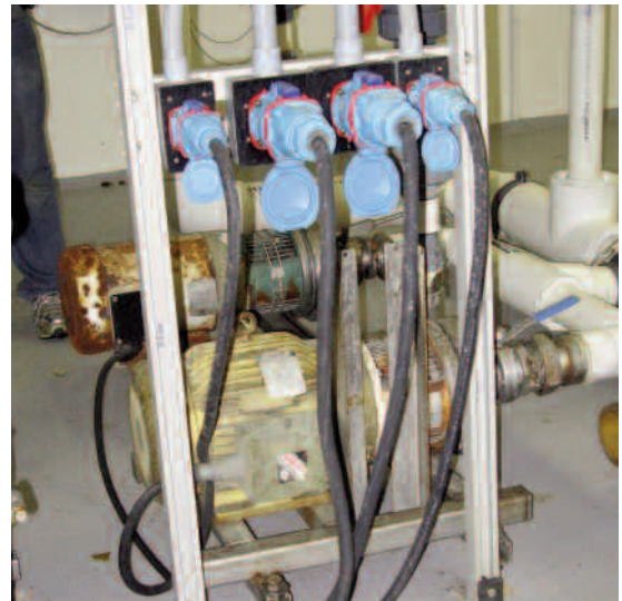
Four Deconnectors provide power to individual pumps used to empty the holding tanks that hold four separate sizes of pickles.
