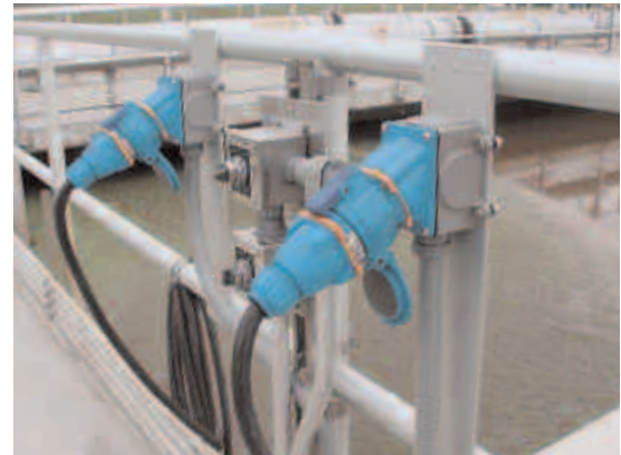
Closeup shows Meltric Decontactors for two adjacent mixers. Pressing the pawl on top of the device disconnects the power safely before the plug and receptacle can be separated.
