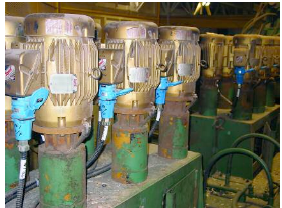
Optimil sawbox at Canfor's Houston, BC mill has 12 motors that must be removed frequently to facilitate routine maintenance. Meltric's switch rated Decontactors (in blue) make the job faster and easier than rewiring each time.
